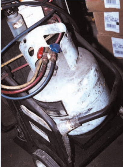
Figure 9: This tank was simply placed on the scale, but not in the retaining ring. The tank is tilted against the side and the scale cannot register accurately, so charging weight may be incorrect.
