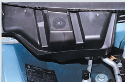
Figure 17: Plastic shield at the fresh air intake of a VW Passat. With an intake air screen above it (not shown) and this cover itself, you'd think the cabin air filter underneath was well isolated from anything but the finest airborne dust.
