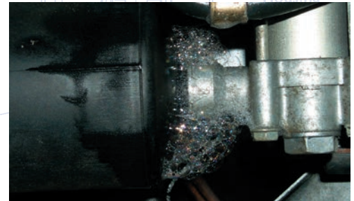
Figure 12 Air Leak Soap Bubbles
