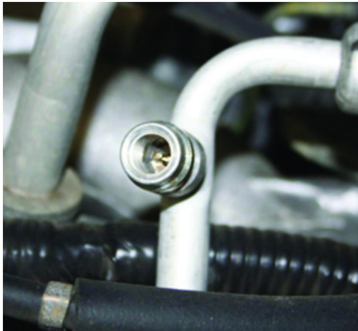
A missing service valve cap can be the source of a small refrigerant leak. The cap contains a seal to help keep refrigerant from leaking.
