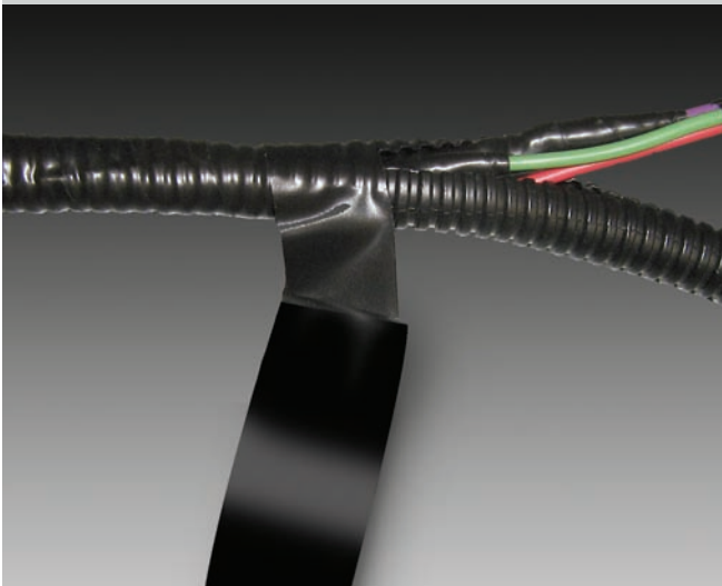
Use flex conduit to protect wiring
