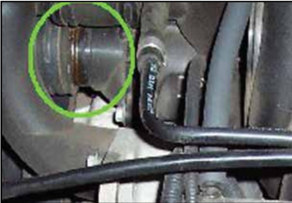
Figure 12: This upper radiator hose is nearly ready to blow off of its fitting.
