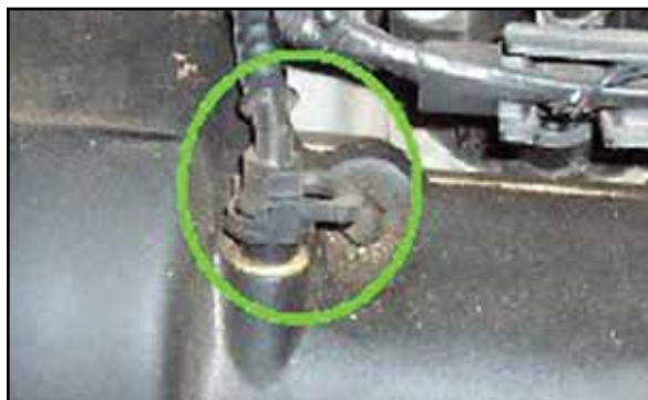
Figure 18: The part-loaded breather fitting is prone to sludge build-up.
