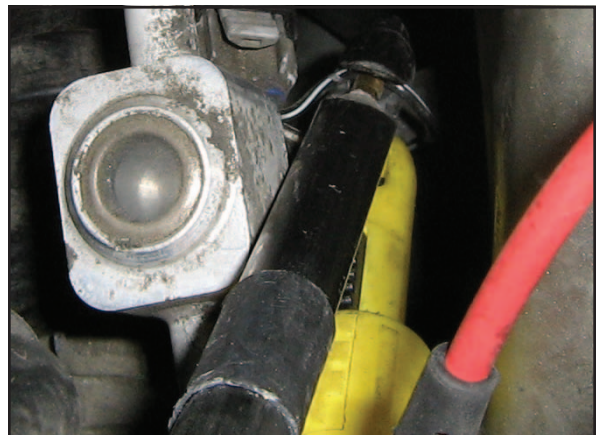
Use a seam splitter to slit the protective sheath, and then use piercing probes to check voltage.
