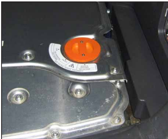
Figure 4: I walked over to the rear of the vehicle to check the battery disable plug located in the rear compartment
