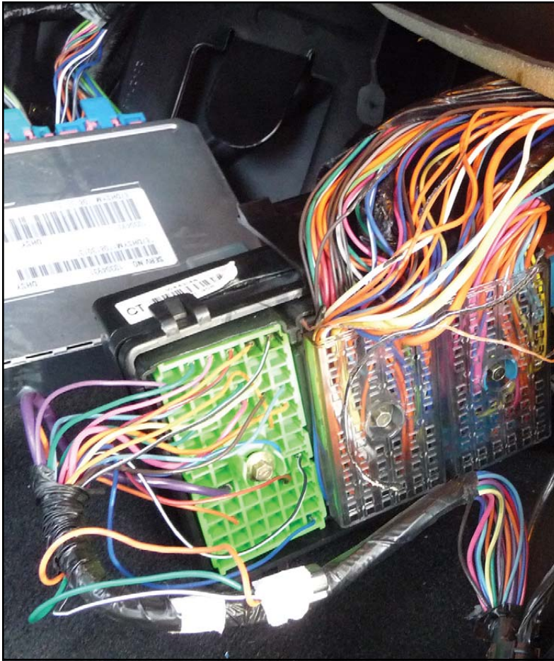
Figure 11: A closer inspection here showed a 12-volt feed line next to the RCDL ground.
