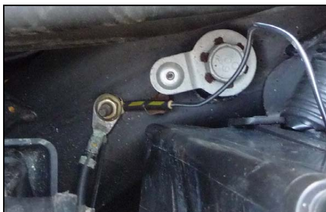
Figure 10: Following the ground wire back through the vehicle, it led me to a junction block in the right kick panel.
