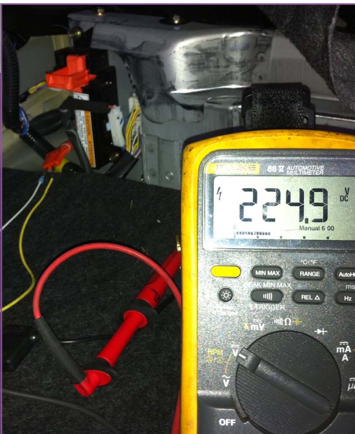
When the reading is positive, the meter is hooked up correctly. Don't make the connection with a live circuit! Disconnect the service plug before connecting your meter, then plug it back in to take the reading.
