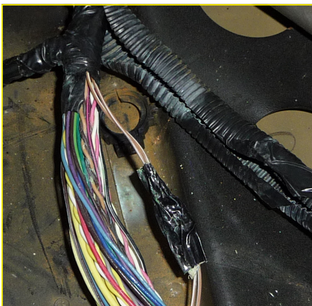
Figure 6: Located a conduit that held the splice internally wrapped with black electrical tape.
