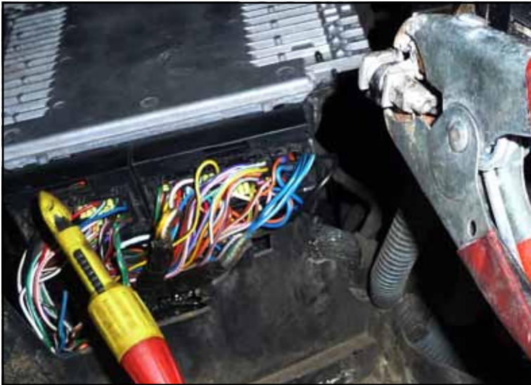
Figure 8: APP Sensor #1 Ref Voltage circuit cut-Short remains.
