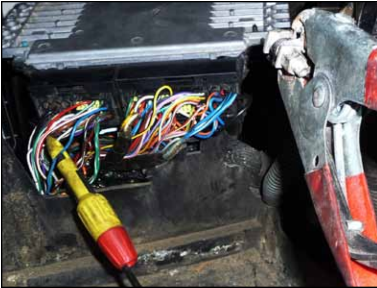
Figure 7: APP Sensor #1 Ref Voltage circuit shorted to ground.
