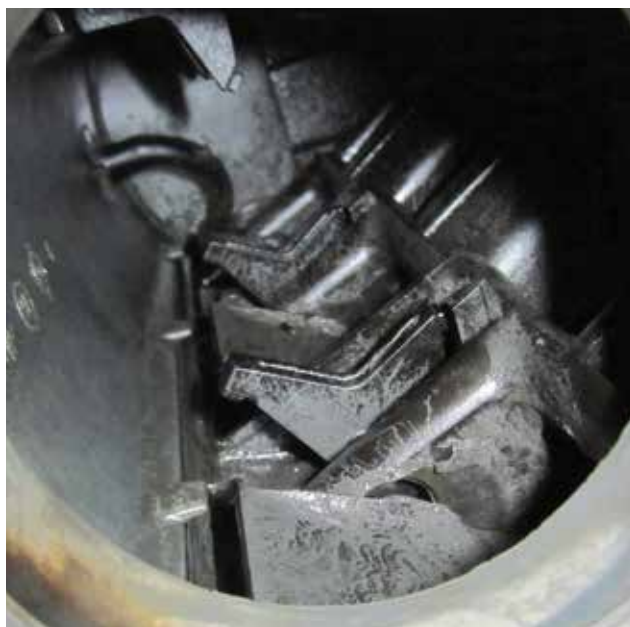
Looking inside this manifold, you can see the coked-up variable flaps, and also the vacuum line at the back coming from the internal reservoir.
