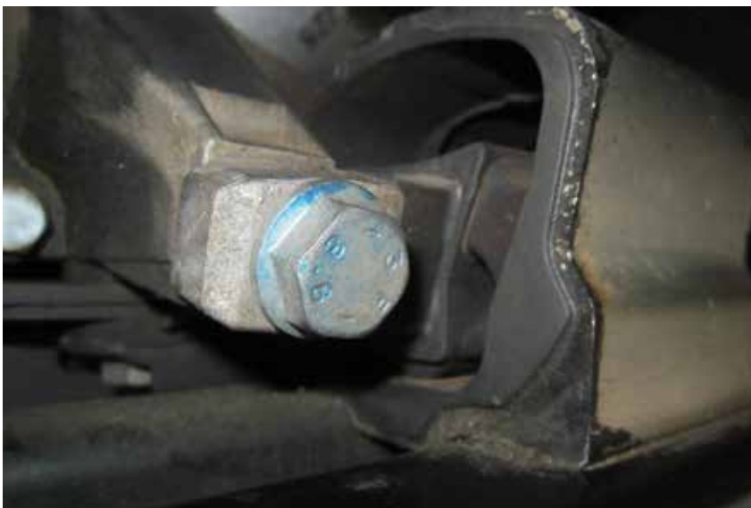
A collapsed transmission mount still in the car. This 2007 E320 had driveline vibration above 40 mph.
