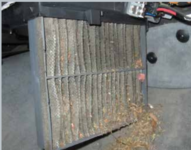
This is the result of poor maintenance -- a clogged filter with mold growth. This vehicle had both low airflow and a bad smell.
