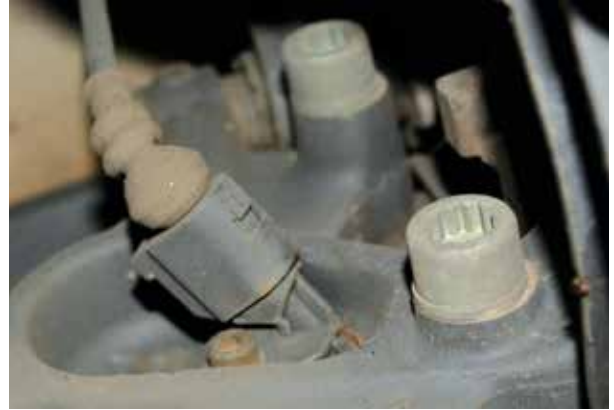
Corrosion around the base of the wheel speed sensor and its bolt can alter the sensor position, changing the air gap between the sensor and tone wheel and reducing the accuracy of the voltage signal to the ABS controller. If the sensor is undamaged, you may be able to remove it (be gentle with its plastic housing), clean the corrosion off of the mounting area, coat it to minimize future corrosion, and re-install the sensor. VW recommends using hot bolt paste (VW part number G 052 112 A3) on the mounting area for Jetta wheel speed sensors, but you should check your repair information for sealer recommendations for specific year and model vehicles.
