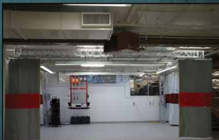
ALUMINUM CLEAN ROOM
