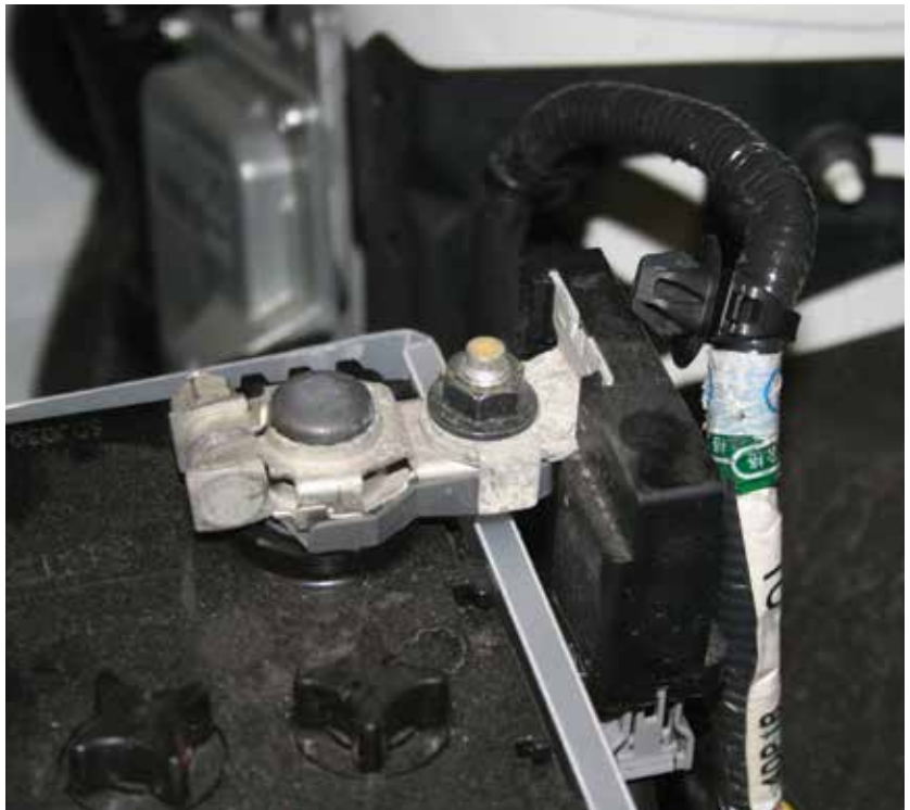
Check the negative battery cable for damage.
