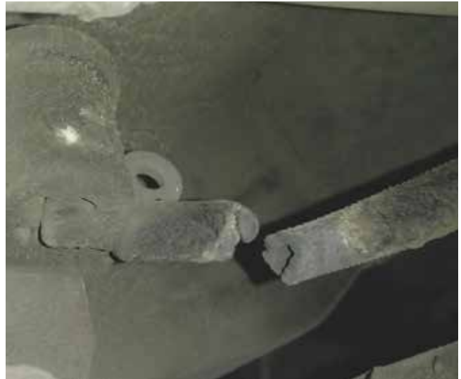
Cracked hose at roll over valve.
