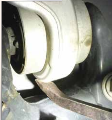
Using light pressure on the bushing with a pry bar can help determine if the bushing has failed.
