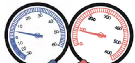
Low pressure switch faulty
