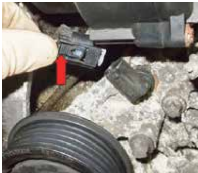
Be sure to check for corrosion on connectors.
