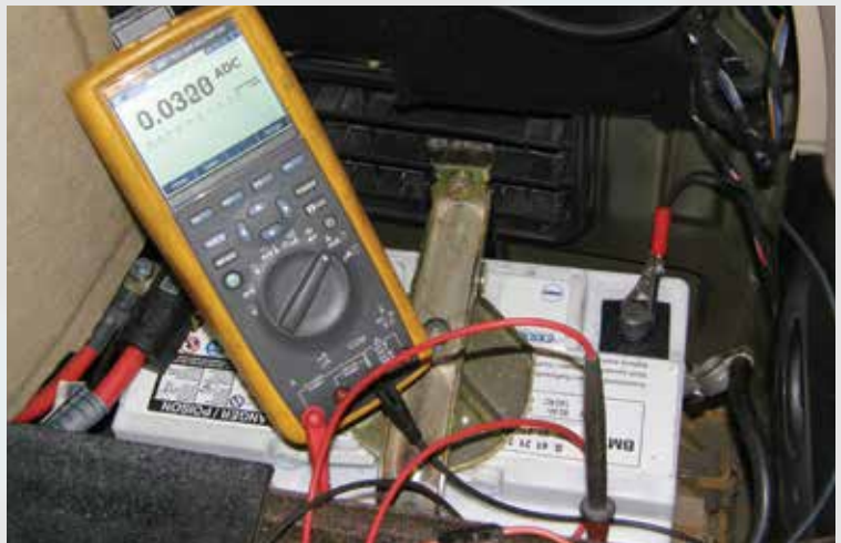
Note the meter is hooked up between the negative battery post and ground.
