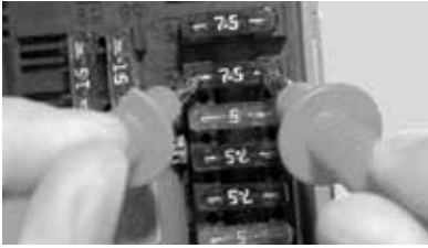
Perform a voltage drop test of the SAM and controllers.
