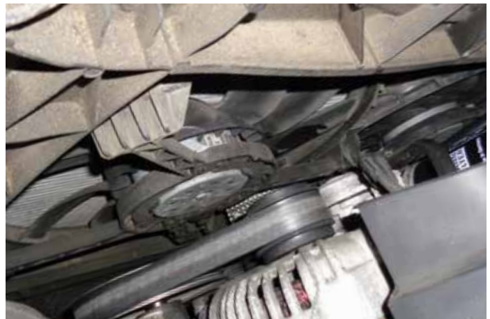
Both fans must work properly for effective A/C operation!
