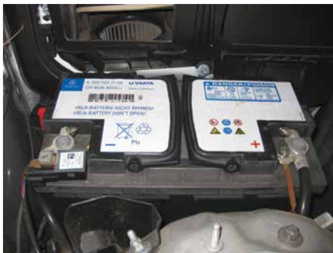
Note the amp hour rating and the IBS at the negative cable of this Mercedes-Benz battery.
