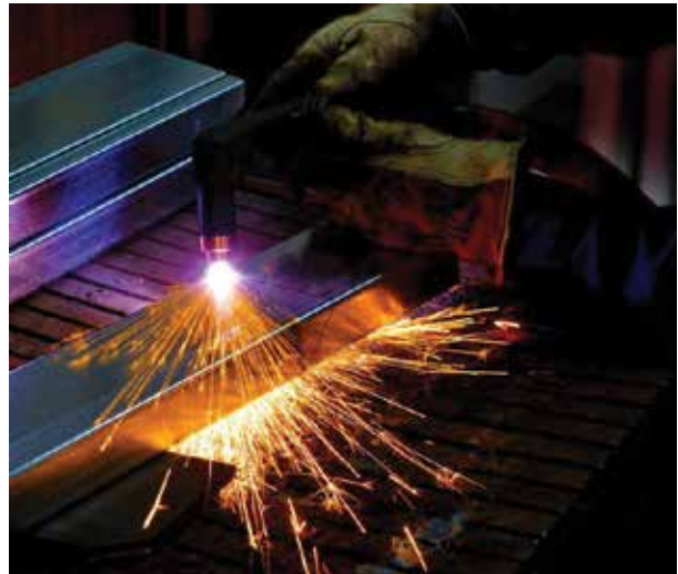
Great welds make solid repairs that usually are at least as strong as the sheet metal around them.
