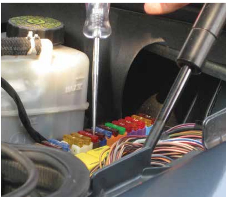
Avoid frustration and embarrassment by checking all the fuses early on!
