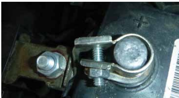
Cheap battery terminals are readily available and often installed poorly. Just because a cable end is new doesn't mean it was installed right or that the battery terminal under it was cleaned.
