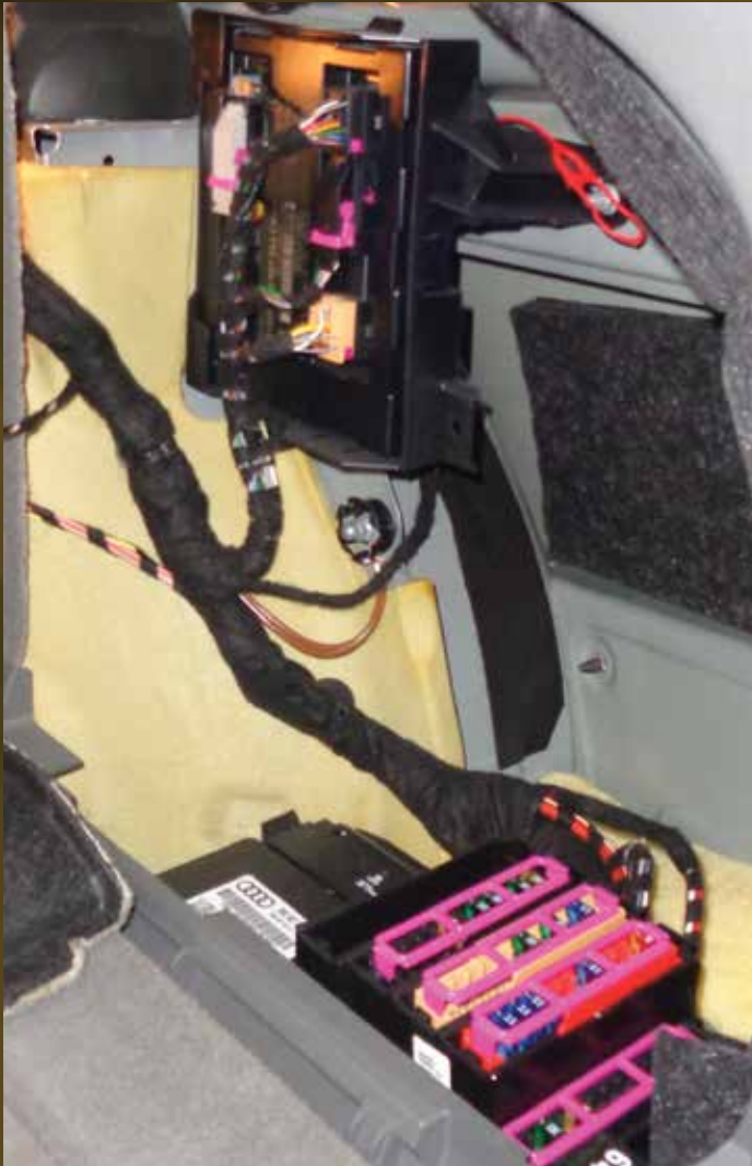
The vehicle battery and primary body control module are located in the right rear corner on this 2012 A4 Avant.
