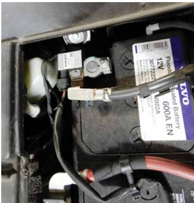
BMS sensor at negative battery cable
