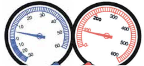
Low pressure switch faulty
