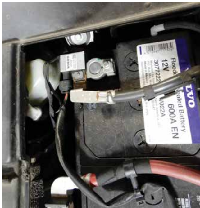
BMS sensor at negative battery cable
