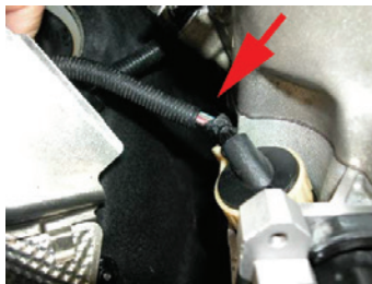
This harness is under tension and has damaged the electrical connector. After replacing the connector, re-route the wires to be completely tension-free.
